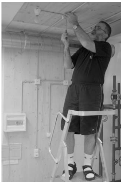
Fig. 9 – Work station for electro-installation.
