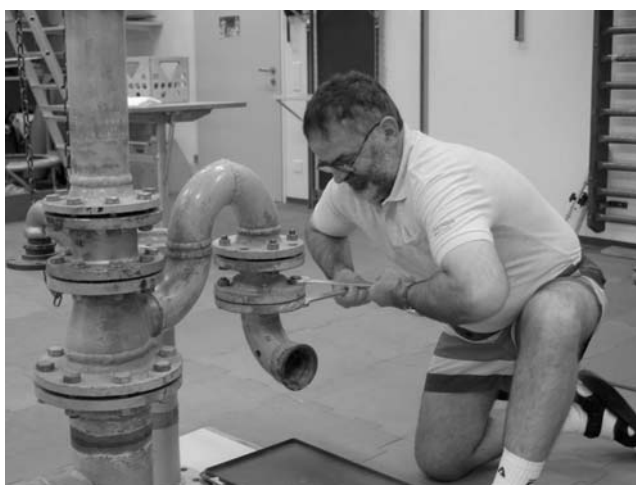
Fig. 8 – For work simulation training, inexpensive devices can be used (assembly system of old tubes).
