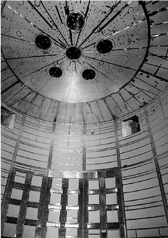
Fig. 16.18 Inside of an industrial spray dryer with atomisation units at the top and explosion venting panels at the spray chamber wall (courtesy of Carlisle Processing Systems – Friesland).
